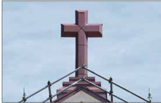
A new cross features at each end of the restrengthened Cathedral roof.
