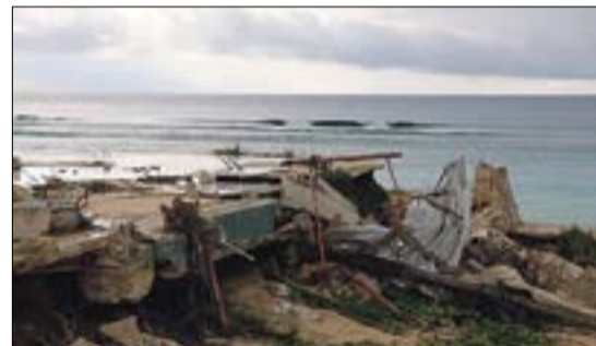
Destruction of buildings on the Western coast of the main island Tongatapu. Photo: Supplied
